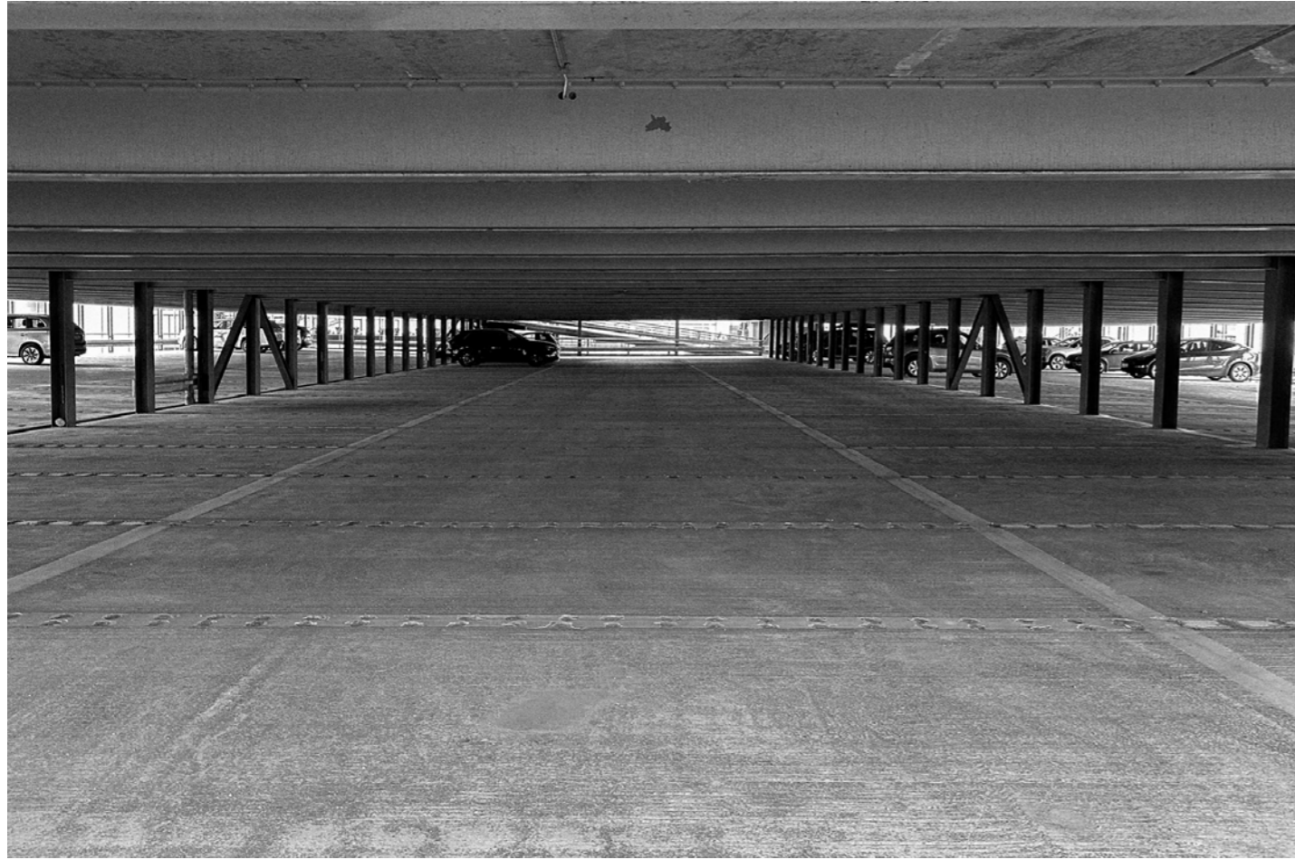
The reduced height on the first floor creates a sense of compression within the space.
